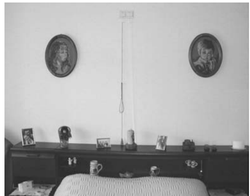
Figure 10. Two bed cords too close to each other: one for active alarm, one to switch off the lights
