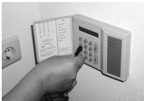
Figure 3. The tenant switches intruder alarm on / off via proximity key
