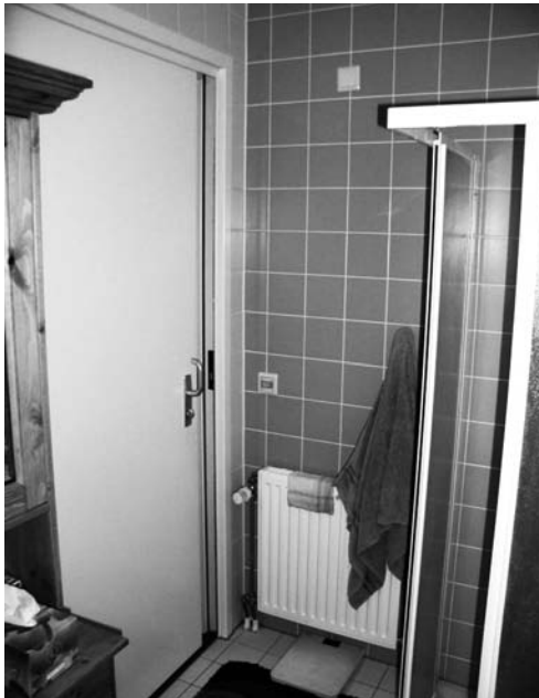
Figure 7. Passive infrared sensor in the bathroom for automatic light
