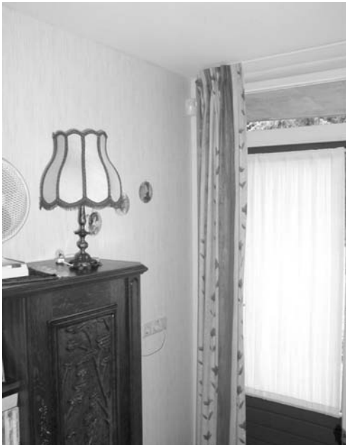
Figure 9. Poorly mounted passive infrared sensor close to and often behind the curtains
